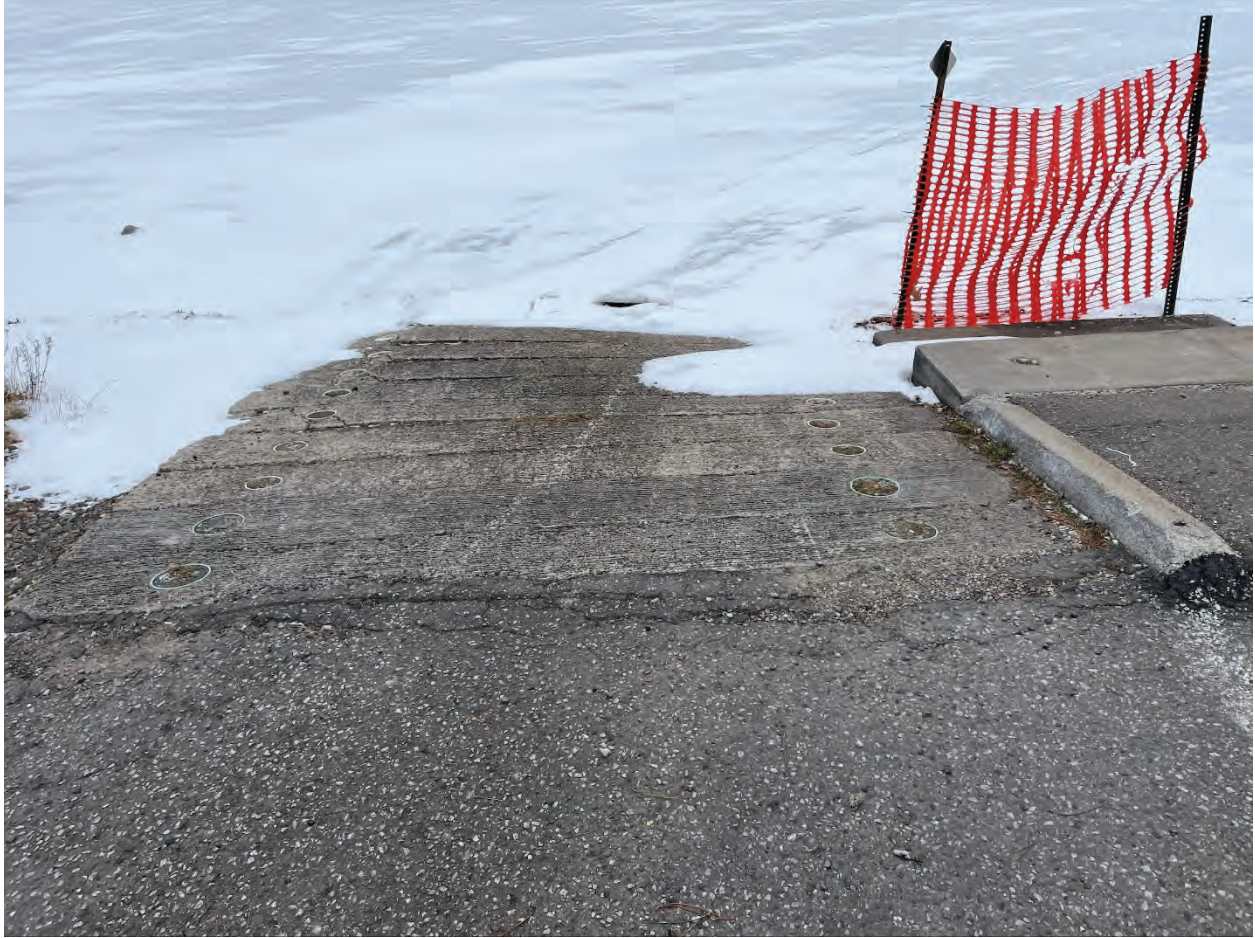
Figure 2 - Lake Lucerne PA boat ramp condition in February 2024
