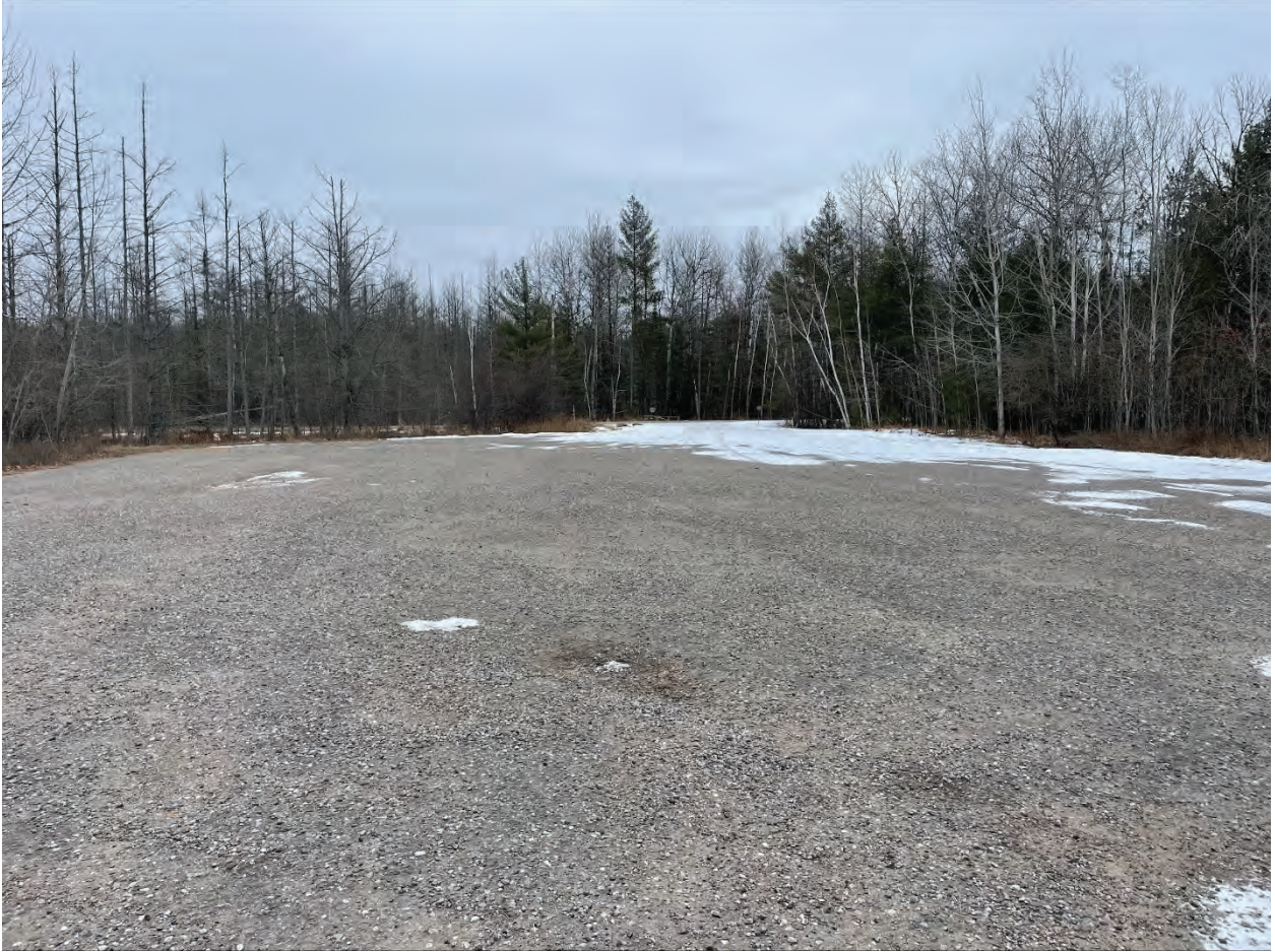
Figure 3 - Lake Lucerne PA pavement condition in February 2024
